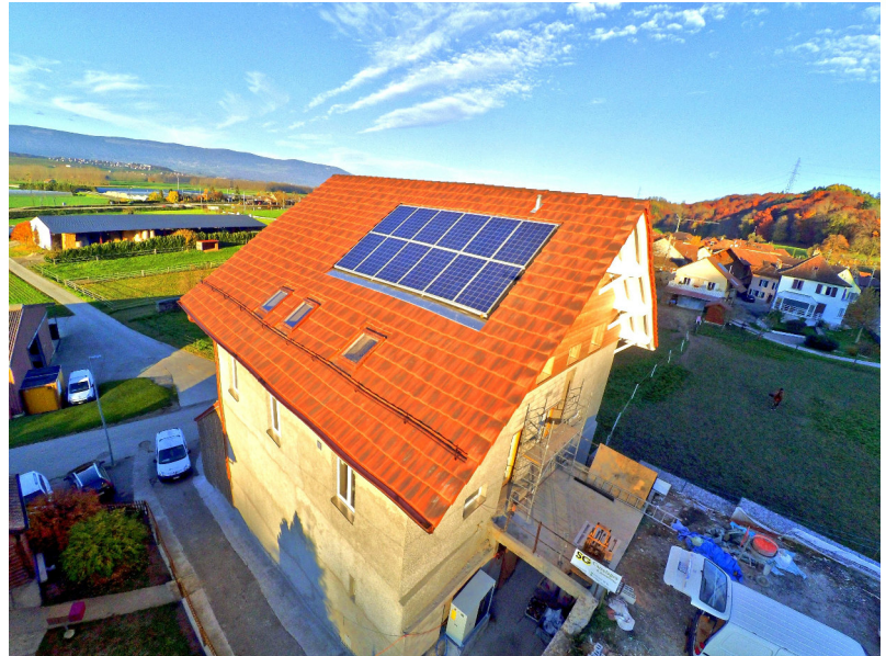
Installation OptiMix maxi 13 kW
